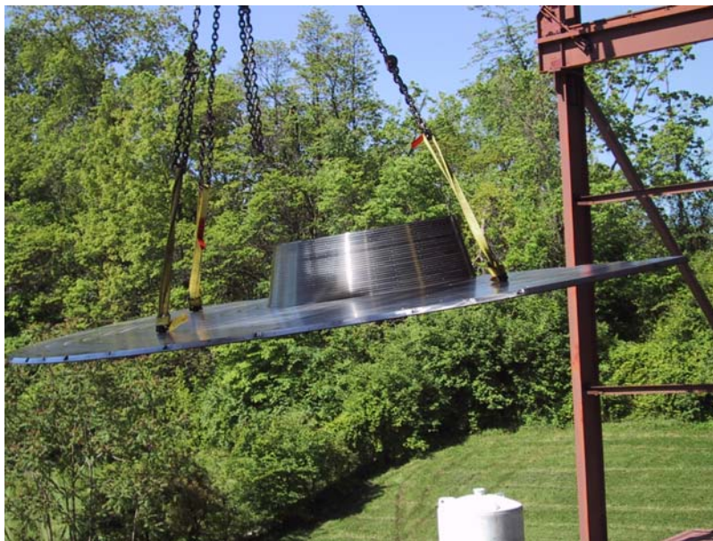
Fig. 1 The mechanical structure for the first (lower) half of the STAR endcap electromagnetic calorimeter as it is craned into the Cooler building for assembly.
